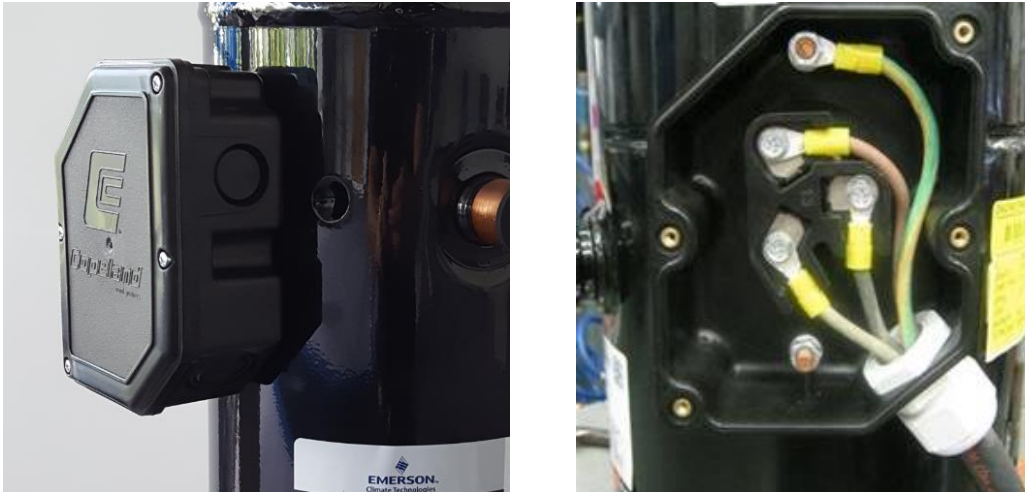
Figure 16: IP54 T-Box and correct electrical installation with cable gland
